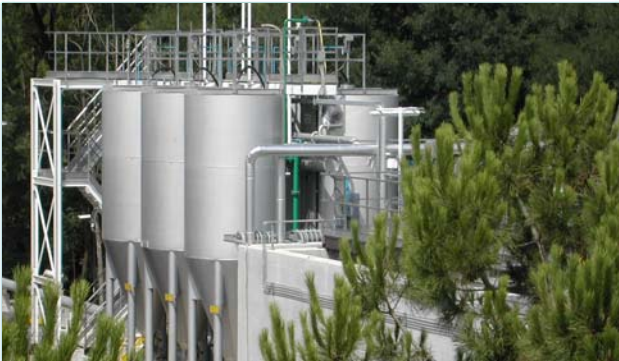
Tertiary filtration plant
